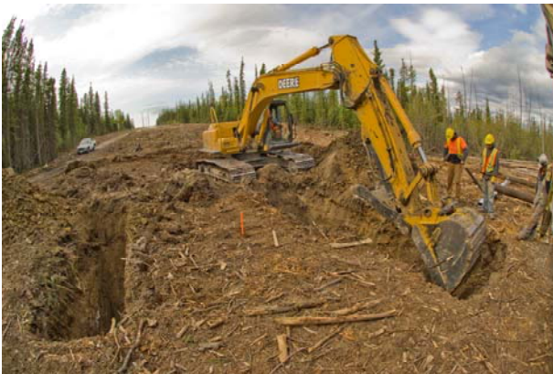
Digging holes for the transmission poles. (L-R) William Fairclough of Carmacks, Tyler Skookum of Carmacks and Gene Hellman. Photo: www.archbould.com
