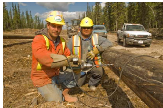
Fred Harper from Pelly Crossing (right) and Jason Rideout, assembling the transmission line structures. Photo: www.archbould.com
