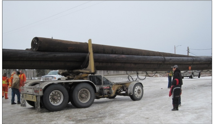
Transporting power poles to the Carmacks-Stewart line construction site. Photo: Yukon Energy
