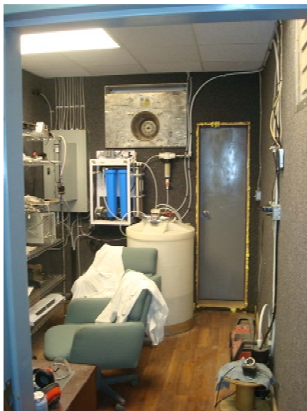
Figure E3: Control Room and Water Treatment Area
