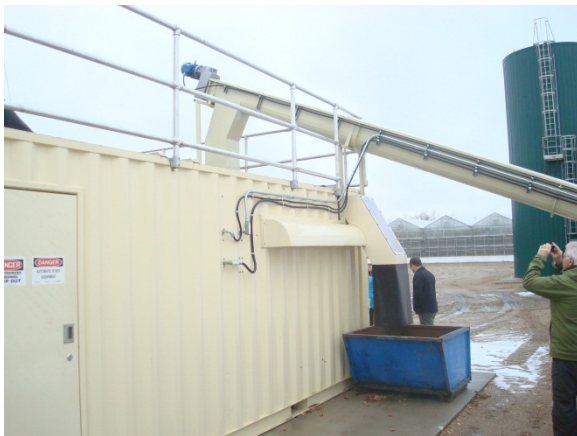
Figure C5: Auger Supplying Biomass
