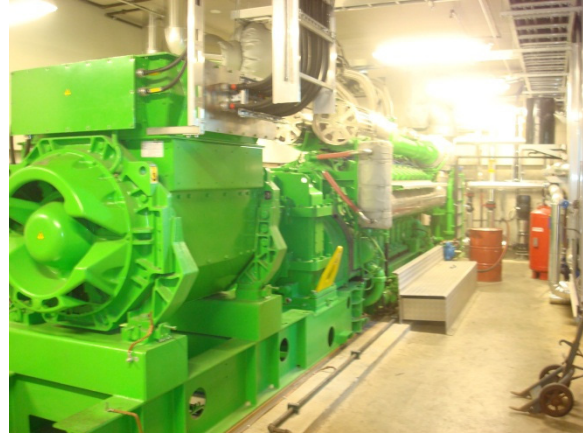
Figure N18: 2 MW e Jenbacher Engine
