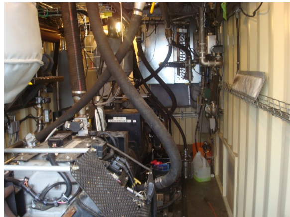
Figure C14: Engine #2 (Rear of Container)
