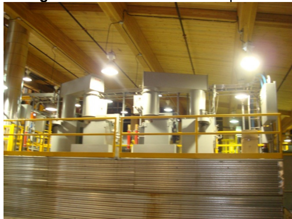
Figure N16: Auxiliary Equipment
