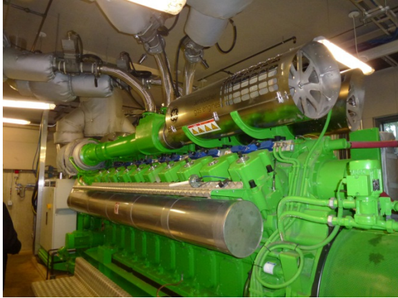
Figure N17: 2 MW e Jenbacher Engine
