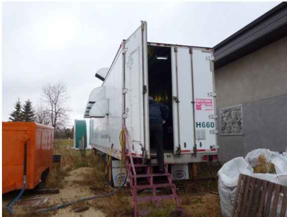
Figure E1: Unit is Located Inside the Trailer
