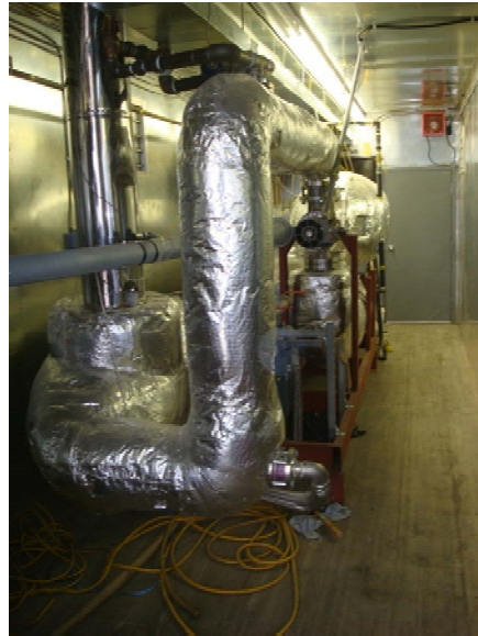
Figure E2: Unit Inside the Trailer
