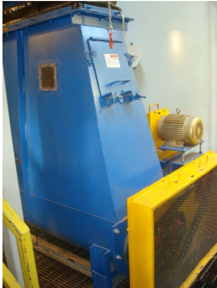
Figure N9: Metering Bin Ahead of Gasifier
